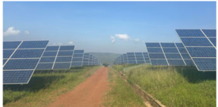
The 28,260-panel solar installation sits on land owned by the Agahozo-Shalom Youth Village.
